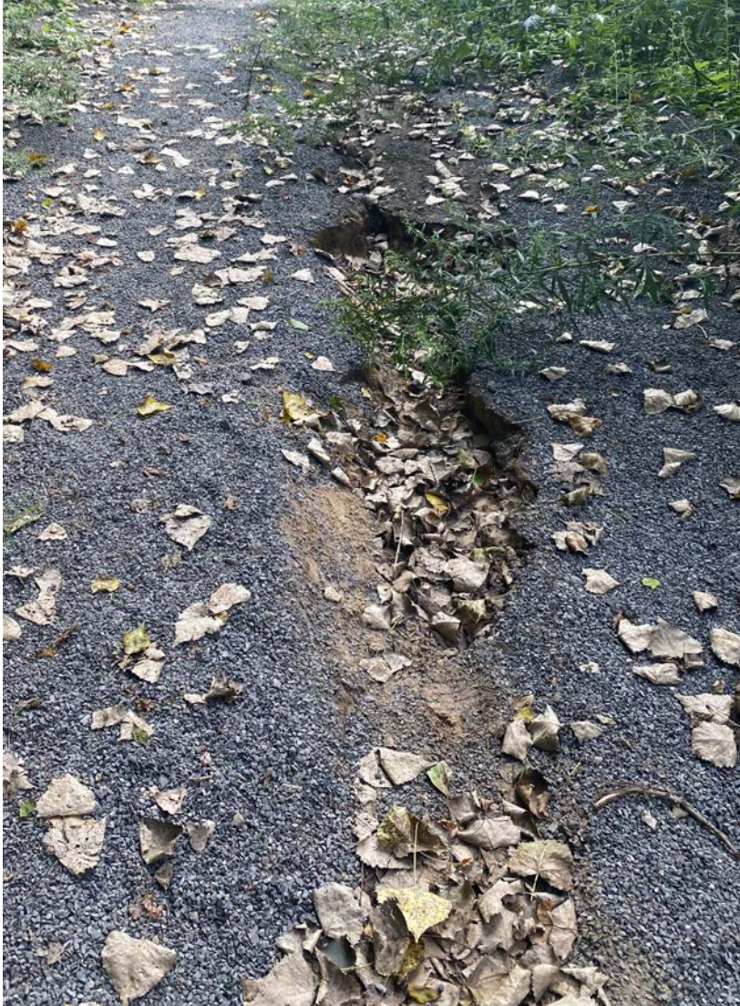
Fig 3a - silt barrier incompletely bisecting the top of the plateau. What is considered dangerous on the right side, if anything?
