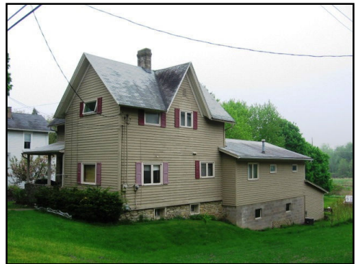
Changing historic features such as the windows can harm the character of the building and neighborhood.
